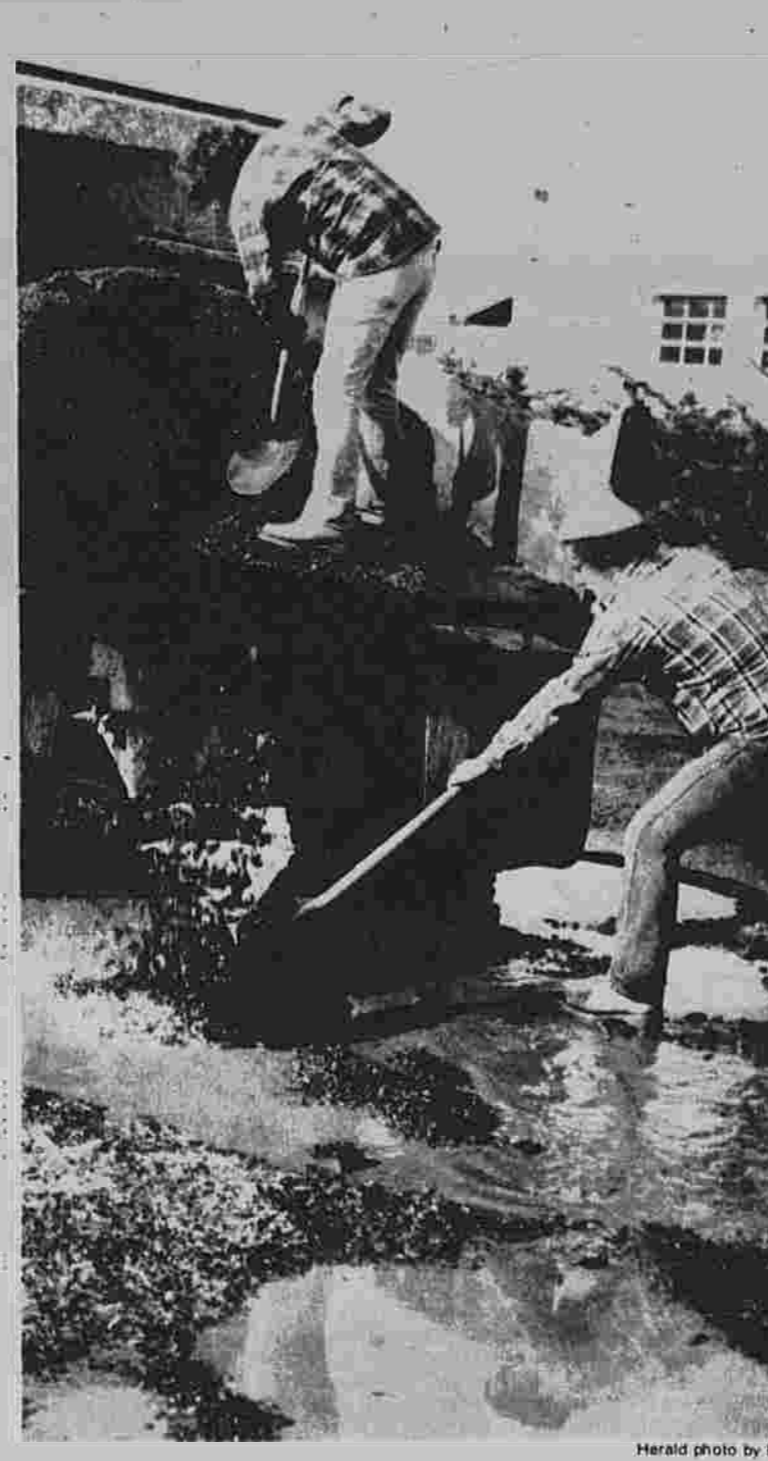
Filling the potholes Ed Bohler (on truck) and George Smith work to fill ruts and potholes in pavement at the Manchester Shopping Parkade. Freezing and thawing have created the annual problem for drivers throughout Manchester.
